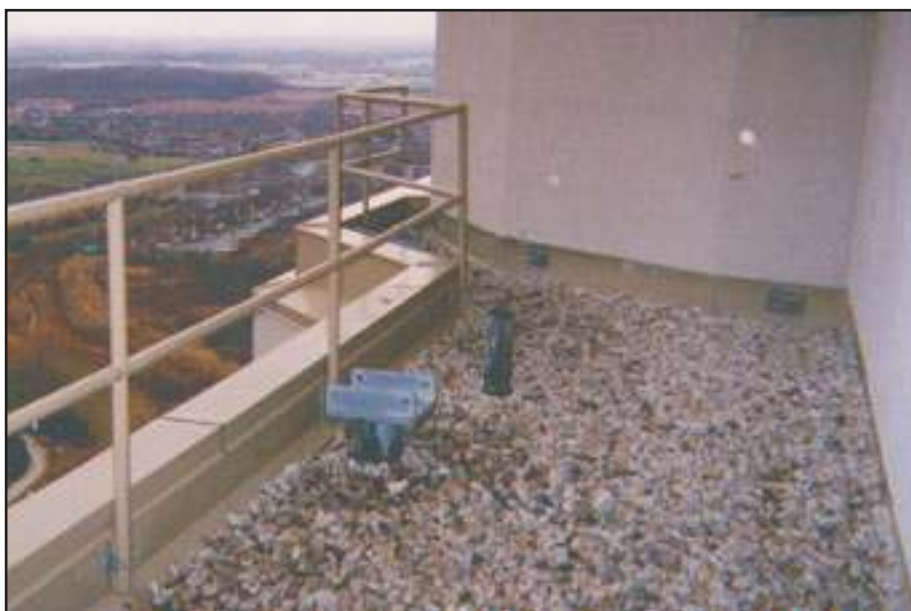
Safety guardrail at davit base anchorage which is used for suspended maintenance. Low parapet requires 42" (1067 mm) high guardrail if workers are approaching within 6'-0" (1830 mm) of roof edge. This installation is located in a narrow roof area.
