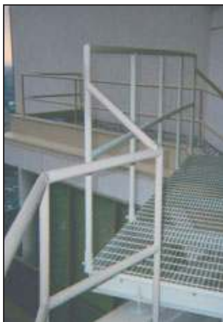
Pro-Bel safety guardrail secured to metal catwalk enclosing narrow roof.
