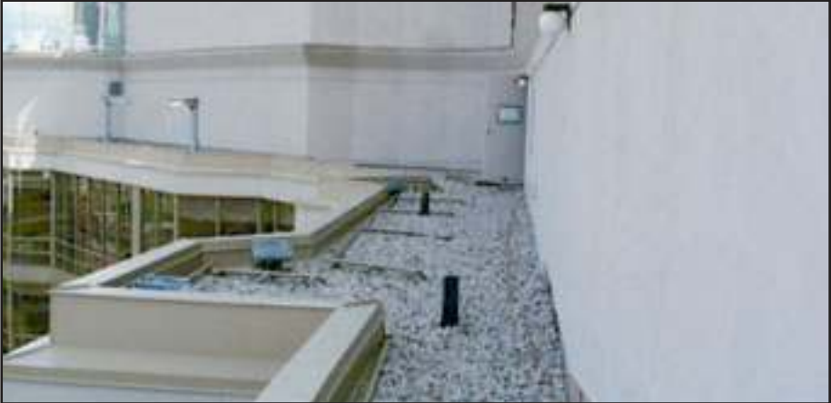
Narrow roof is being retrofitted with Pro-Bel safety railing. Vertical posts are being laid out and prepared for installation to inside of parapet wall.
