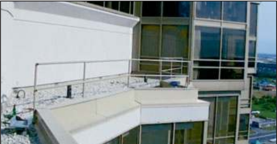
The angular roof line required complete perimeter protection. This Photo shows partial installation of Pro-Bel safety railing.
