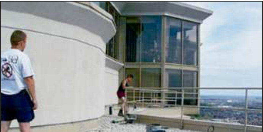
Pro-Bel installers adjust corners and horizontal top rail to ensure guardrail is level and square before tightening up vertical posts.
