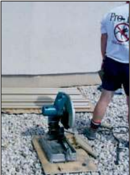
Pro-Bel installers cut the horizontal rail on site to length as required.
