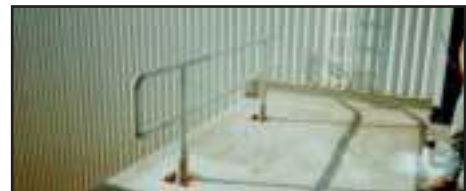
Localized railings provide added protection near access hatches, doors, and/or around mechanical equipment.
