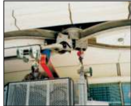
Steel I-beam monorails at turning hub shows battery powered trolleys used for platform “drops” which are plugged into permanent soffit electrical outlets when not in use.
