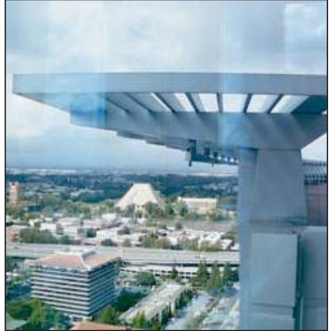
Closeup photo of curved screen canopy showing terminal end of monorail secured to canopy structural supports. Aluminum monorail was factory pre-curved in 12'-0" (3.7 m) sections prior to installation on custom designed hangers.
