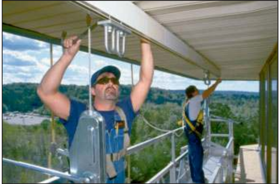
Workers adjusting new Pro-Bel exterior monorail system which accommodates four trolleys for a two person platform (two for suspension of the platform and two for worker's lifelines). Suspension cable is temporarily secured to the structure above the soffit to facilitate installation. Monorail has been powder coated to match soffit finish. Overlook at Great Notch, Little Falls, N.J.
