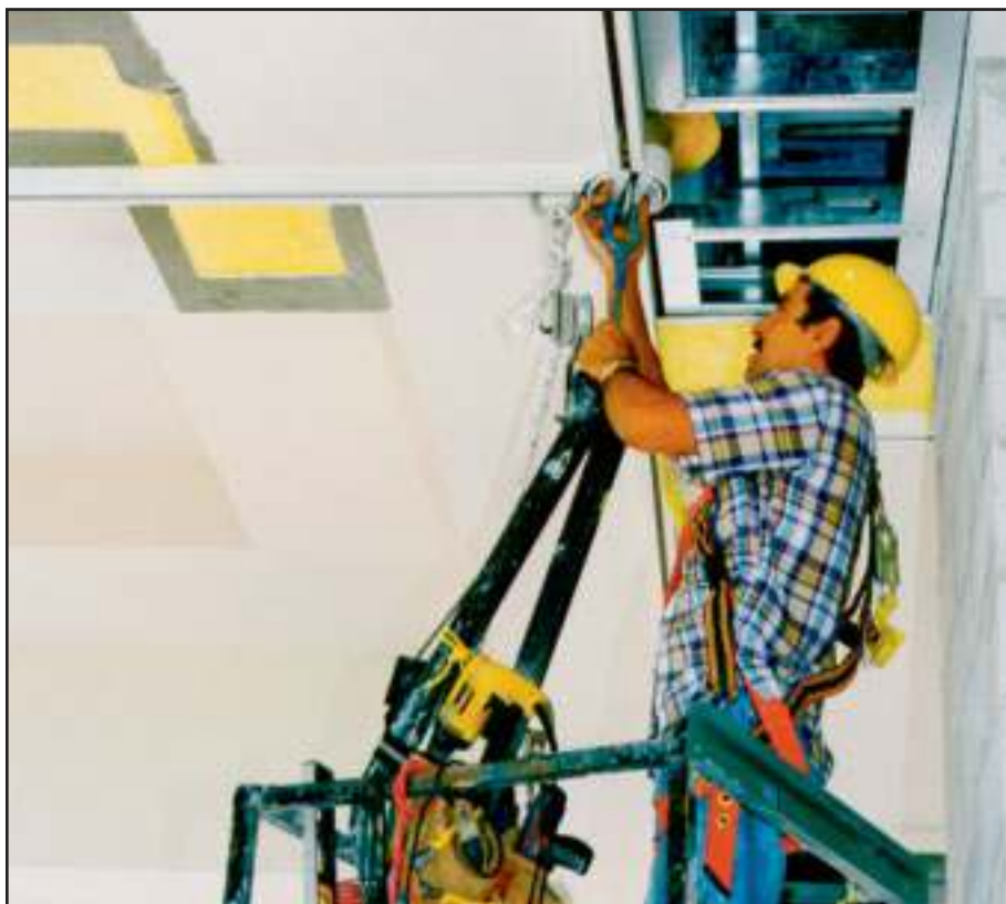
This photo shows worker finishing ceiling around Pro-Bel monorail and corner-turning hub while working from a single work cage. The hub facilitates automatic turning at corners. Diplomat Hotel Resort, Hollywood, Florida.
