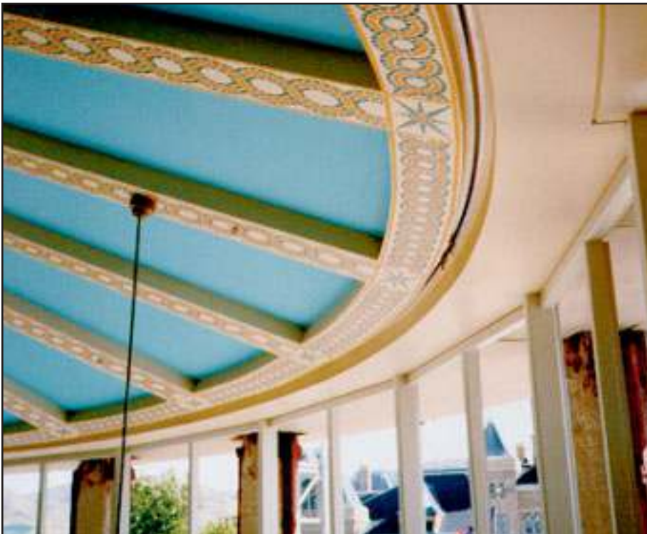
Pro-Bel monorails are often installed in decorative ceilings. This curved monorail forms a complete circle. Salt Lake City Courthouse, Utah.
