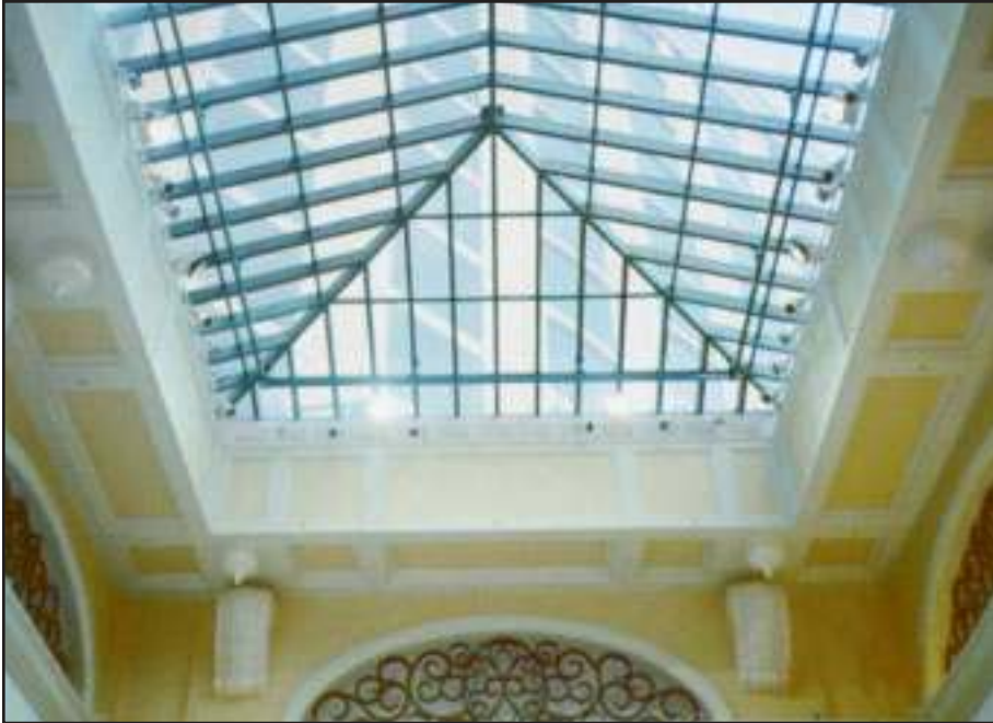
Atrium showing perimeter standard monorail blending in with aluminum clad steel rafters. Separate monorail is located at ridge point. For window cleaning, platform can be suspended at any desired angle or height around all four sides of atrium glass. Beau Rivage Hotel, Biloxi, Mississippi.
