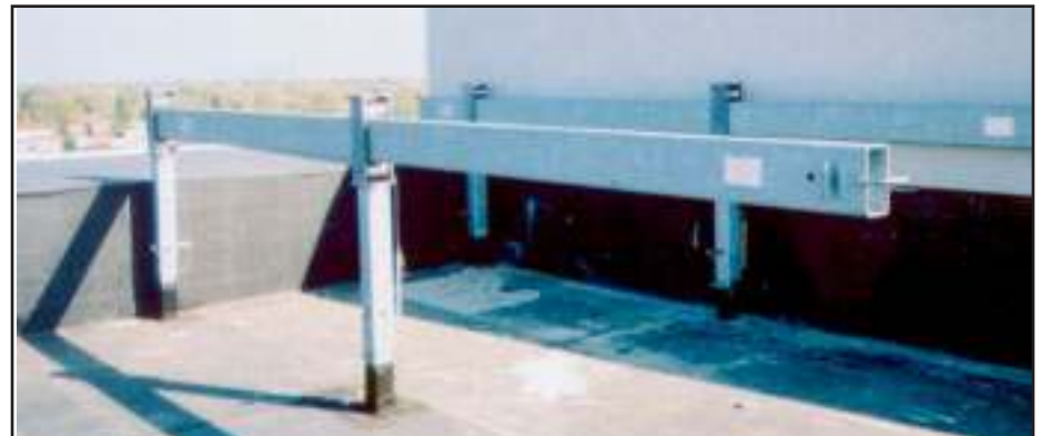
Pro-Bel fixed outrigger beam(s) with sliding beam provides an ideal solution for reaching over wide parapet for ground rigging of platform. Separate lifeline anchors (not shown) are located further back on roof. Amerisuites Hotel, Chicago, Illinois.
