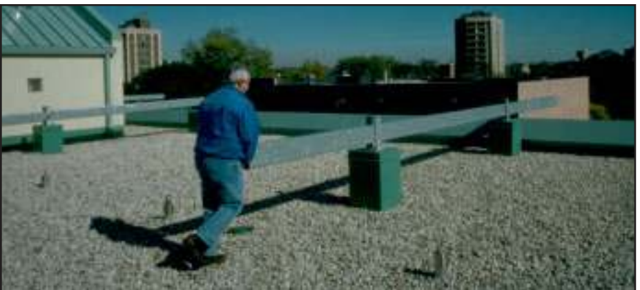
Workman demonstrating how sliding beam is pushed into position (fixed outrigger beam) in preparation for window cleaning operations using a platform.
