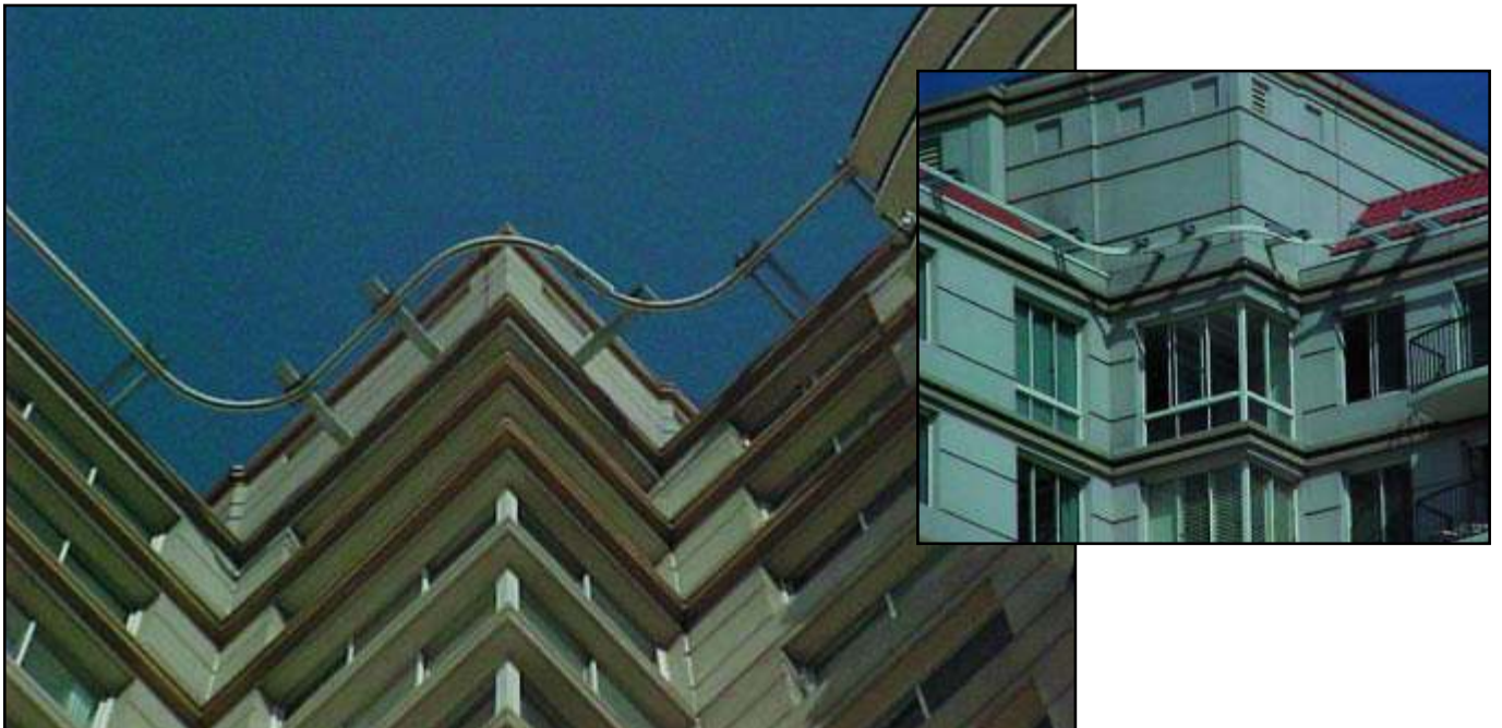
Pro-Bel aluminum "Halo" monorail provides continuous support for a suspended platform around most of this highrise apartment building, with davits serving the remainder of building. In addition to being functional, the "Halo" adds a certain aesthetic or style to the project. The Pacific Condos, Long Beach, California.
