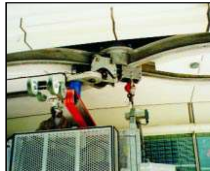
Steel I-beam monorails at turning hub shows battery powered trolleys used for platform “drops” which are plugged into permanent soffit electrical outlets when not in use.
