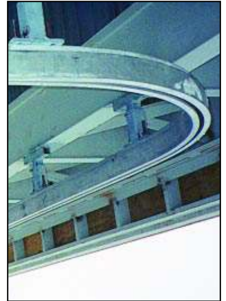
Close-up construction photo of curved monorail showing typical securement to building structure and turning radius at corners.
