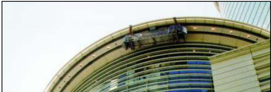
Platform is suspended from trolleys secured to soffit mounted steel I-beam monorail. Recessed facade at upper level requires platform to be switched from an interior monorail to an exterior monorail and vice versa using a turning hub or “turntable” (see close-up photo below, right). Enron Building 2, Houston, Texas.
