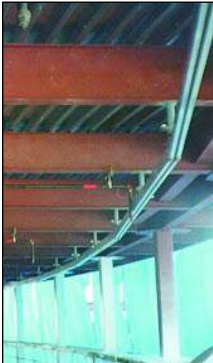
Construction photo shows interior atrium and how segmented monorail is used to provide turning radius for curved building applications (for suspended platform).
